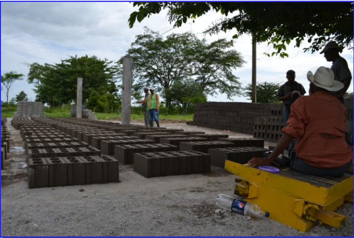
The block factory is just another opportunity for the church to employ the impoverished while also meeting a need for building more houses at Casa Hogar Vida.
